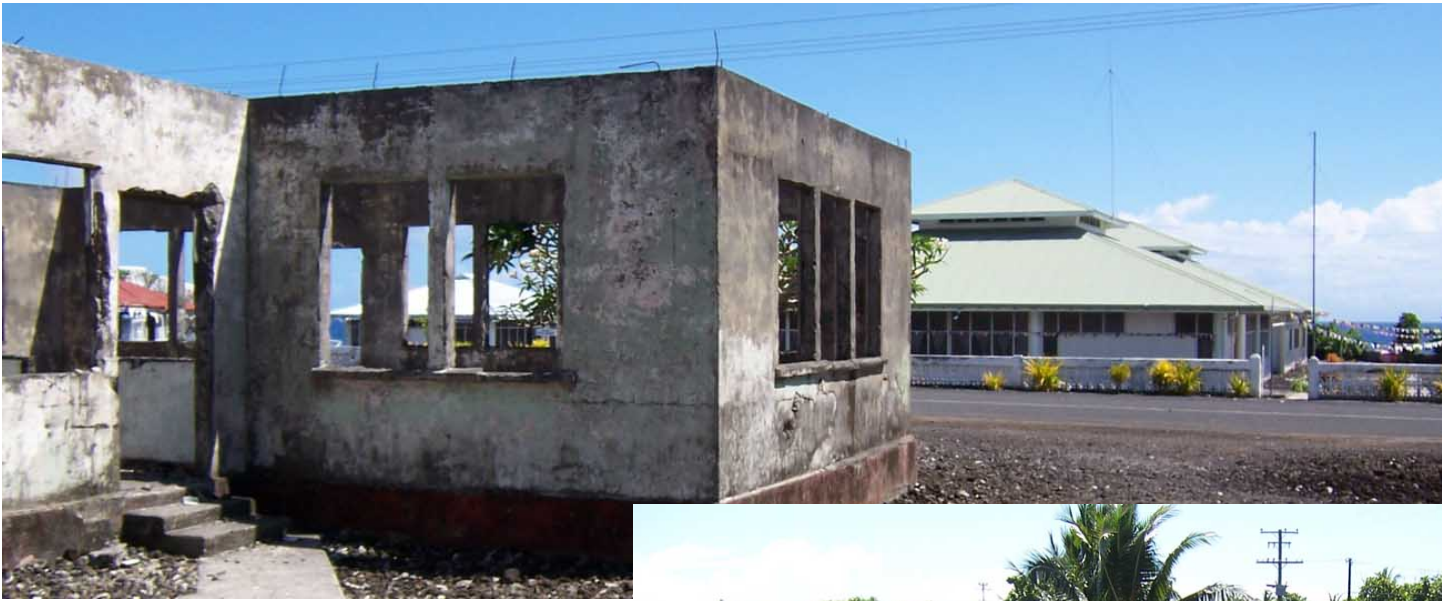
Vacant building across the street from District Hospital
