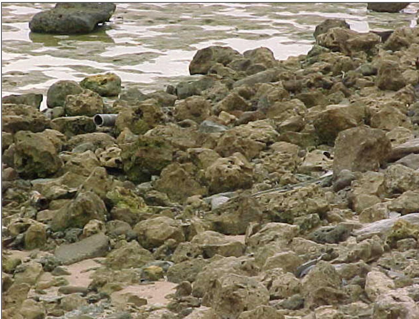
Figure 17. Limestone boulders from failed coastal protection structures.
