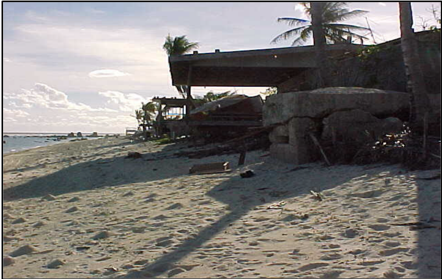
Figure 6. Characteristics of the eroding beach (looking west).
