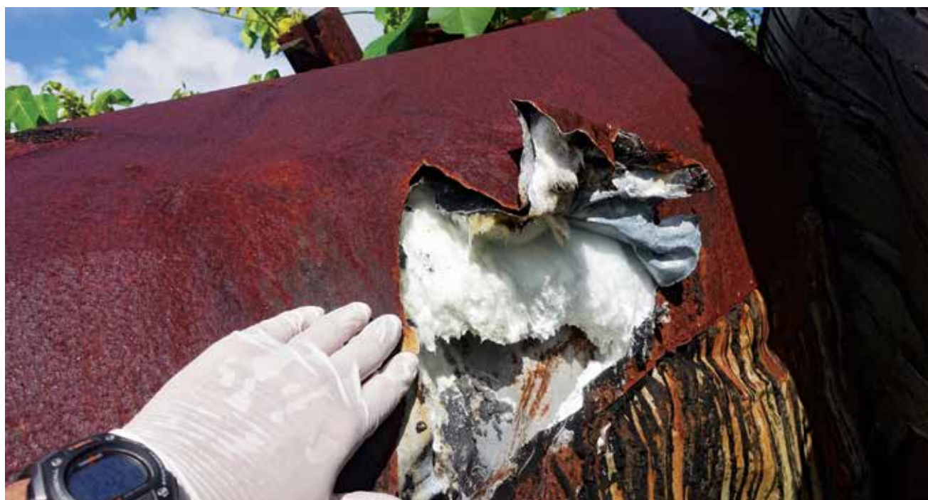
Figure 98: Asbestos that is left exposed can cause serious harm and even death. (PacWastePlus-SPREP 2022).
